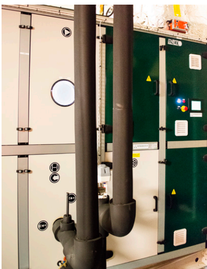
An installed DST Flexisorb dehumidifier in Oasens ice rink ventilation room.
